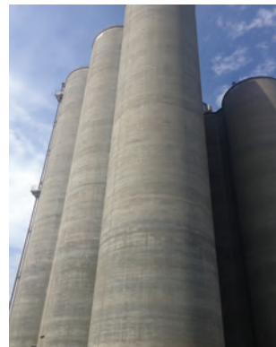
Figure 1-5. Storage silos for cement at a manufacturing plant.
